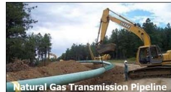
Natural Gas Transmission Pipeline
