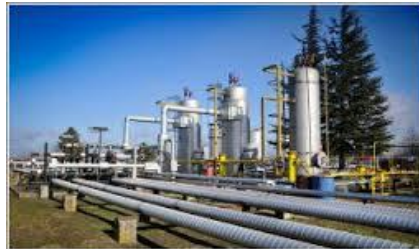
Natural Gas Gathering System
