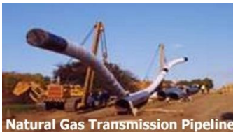
Natural Gas Transmission Pipeline
