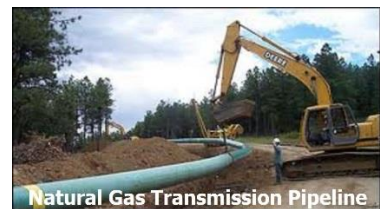
Natural Gas Transmission Pipeline
