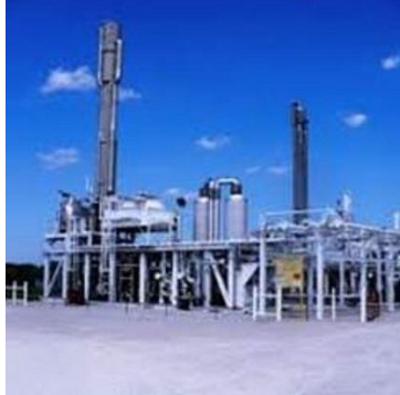
Natural Gas Processing Plant
